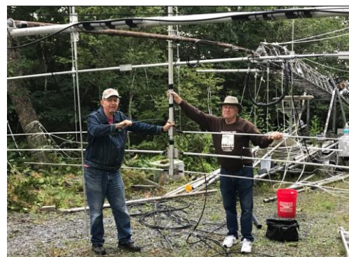
Figure 9. Dick W3OA and Paul W3GQ working on the W4MW 6 meter array
