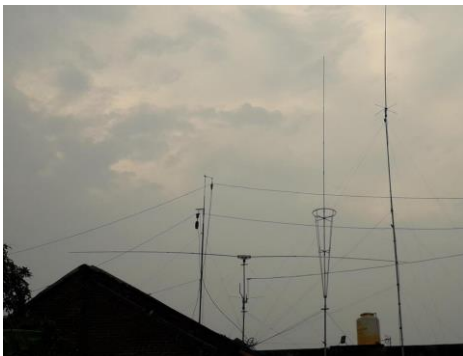
Figure 15. YG3ASG HF and VHF antenna farm
